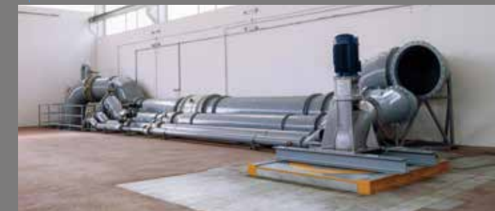
Sala prove Testing Room
