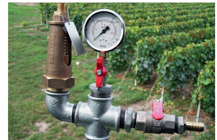
▲ Pressure regulator with safety valve.
